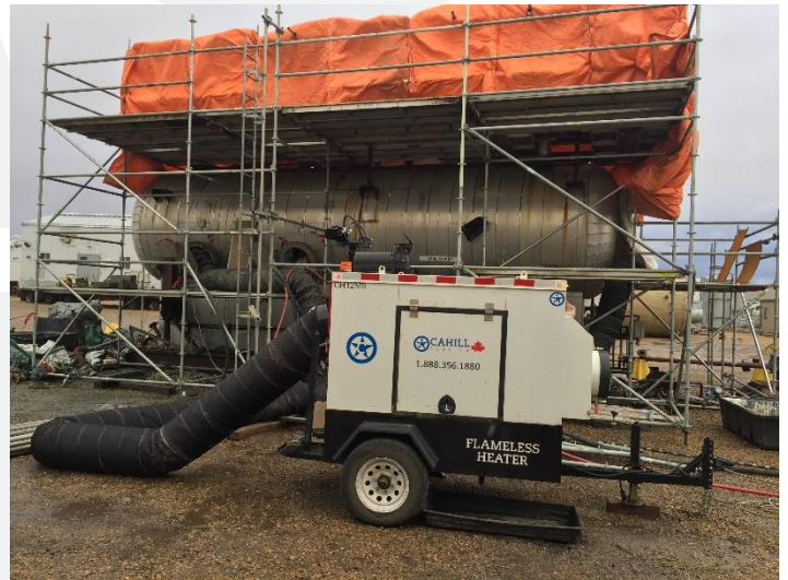
A CH12MS heater thawing critical equipment on an oilfield
