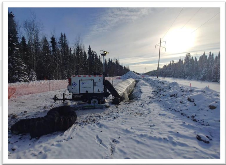
A single CH12MS heater heating a large section of a pipeline in winter conditions
